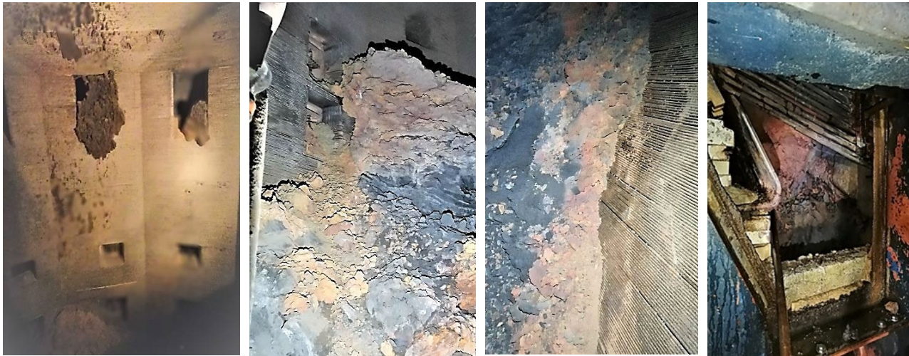
Figure 6. Slagging in the boiler furnace
