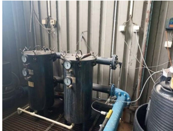
Figure 3. Device for removing iron and adjusting the pH value of returning water in DHP "Krivi Vir" in Niš
