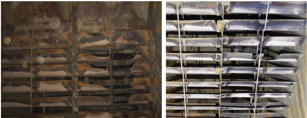
Figure 2. The condition of the turning elements under the rotary air heater
